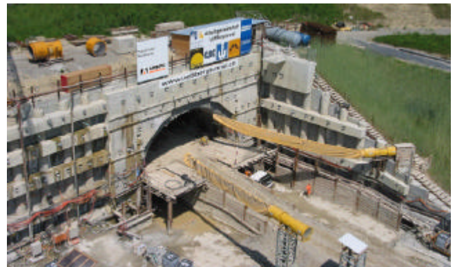
Fig. J: Portal view of the Gänziloo excavation site / driving the Juchegg soft ground section
